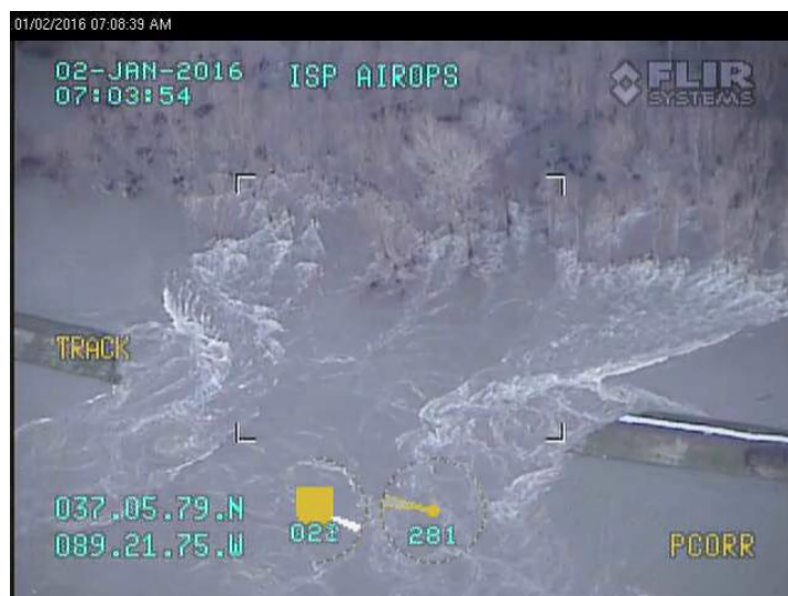
Break in levee during Mississippi River flooding near Miller City, IL, Jan 2016
